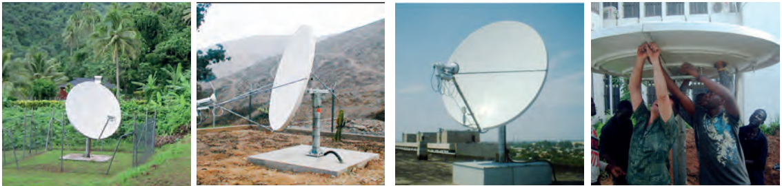
From left to right: GCI satellite terminals at auxiliary seismic station AS24, Rarotonga, Cook Islands; auxiliary seismic station AS78, Nana, Peru; NDC Tashkent, Uzbekistan; setting up the GCI satellite terminal at the NDC in Abuja, Nigeria.
