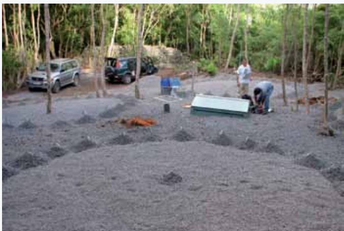
THEME 3. COMPLETION OF SITE PREPARATION FOR INFRASOUND STATION IS42, AZORES, PORTUGAL, AUGUST 2010.
