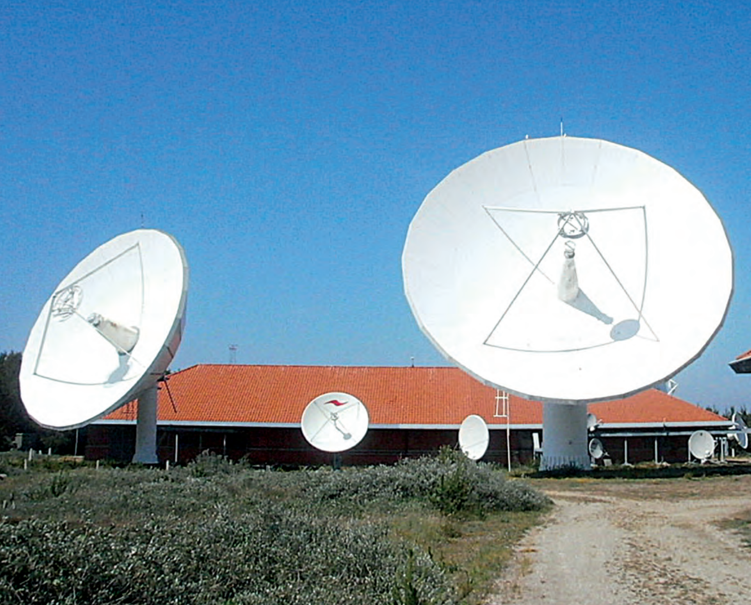
The Global Communication Infrastructure teleport at Blåvand, Denmark
