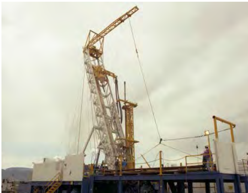
A rotary drill rig, which is capable of drilling to over 1,000 metres depth in all types of formation (alluvial deposits to granite). This is by far the most complex and demanding drill rig.
